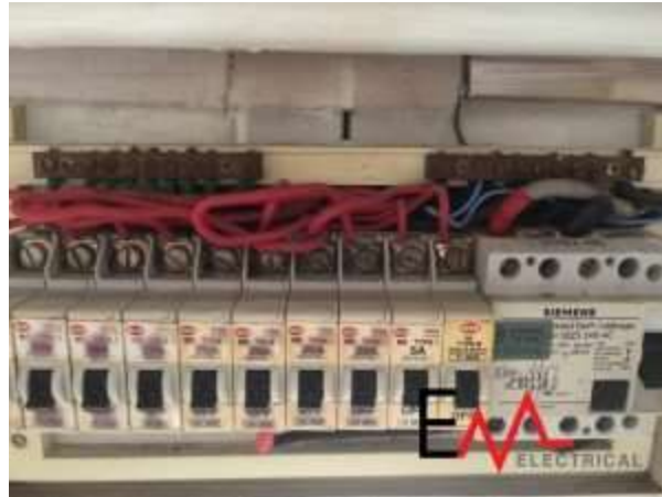
Figure 12. Bad Wiring or loose connections
